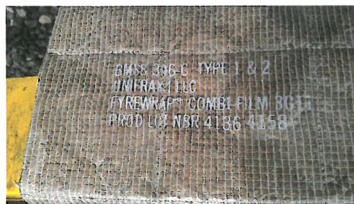
Figure 4 – Fire Blanket Material Used to Wrap the Through-Bolt on the Treated Pole.
